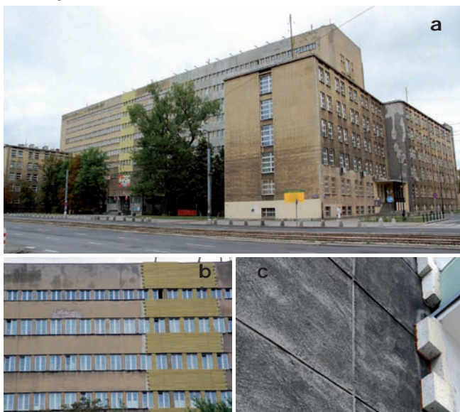
2. Typical process of insulating the elevation using the dry method. Building was originally covered with coarse double-layer plaster with regular geometric divisions made in the top layer - Warsaw, 218 Al. Niepodległości, completed in 1939. 2a. General view of the building; 2b. Fragment of the insulated elevation; 2c. Fragment of the insulation course; visible considerable thickness of the insulating layer and blurring of the wall texture. Photo by J. Lewicki, 2008
