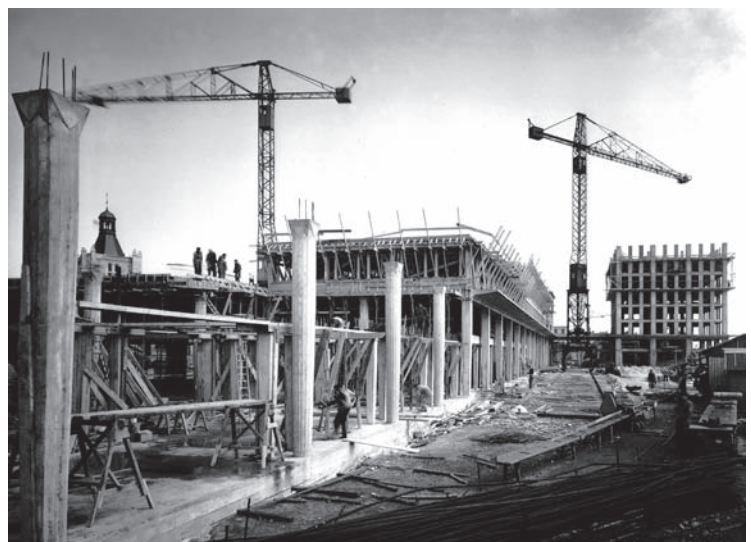
5. Construction works from the side of the sea around 1955. © Robert Lhomme's collections
