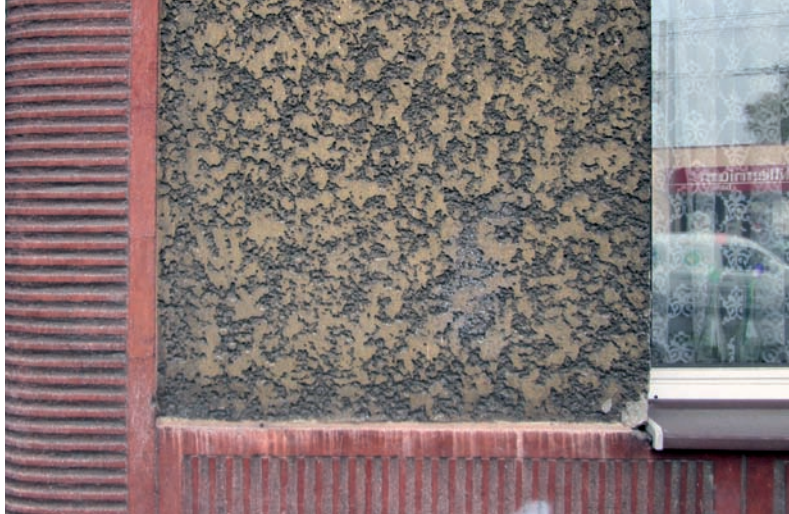
4. Rubbed Tyrolean render in yellow, in composition with red faux stonework render on a building façade at Chylońska 39, Gdynia
