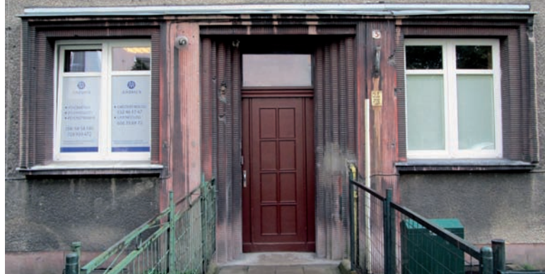
26. Portal at Bema 5; faux stonework finish before restoration
