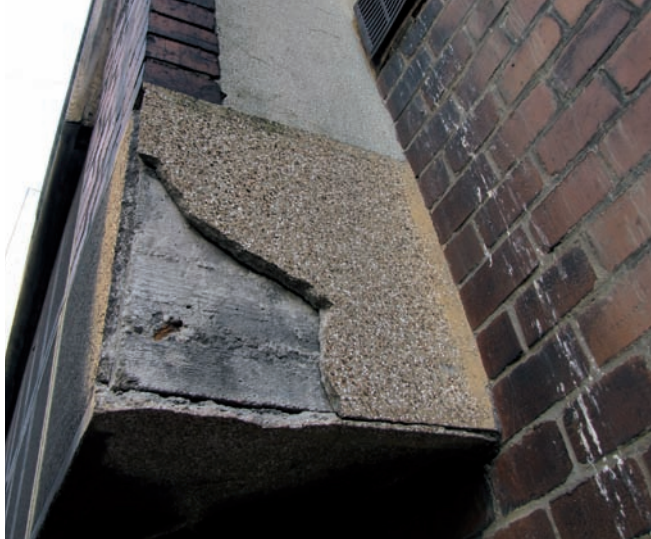
25. Faux stonework finish on a reinforced concrete bay window cantilever, townhouse in Katowice, Stalmacha 23
