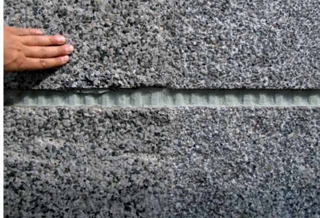
10. Washed render on the townhouse façade at Świętojańska 105, after restoration. Left - original finish, right - reconstructed finish.
