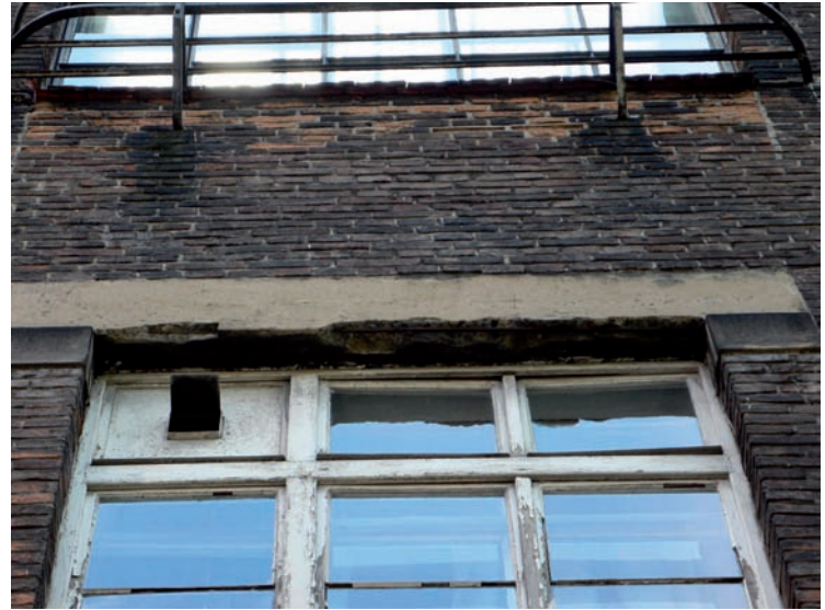
7. Kraków, Academy of Fine Arts Faculty of Industrial Design: rear elevation, detail of the reinforced concrete beam of a window lintel with a visible loss of the concrete covering of a rebar; this might be interpreted as a result of poor workmanship or corrosion caused by the lapse of a hundred years. Photo by W. Affelt (as of June 2009)
