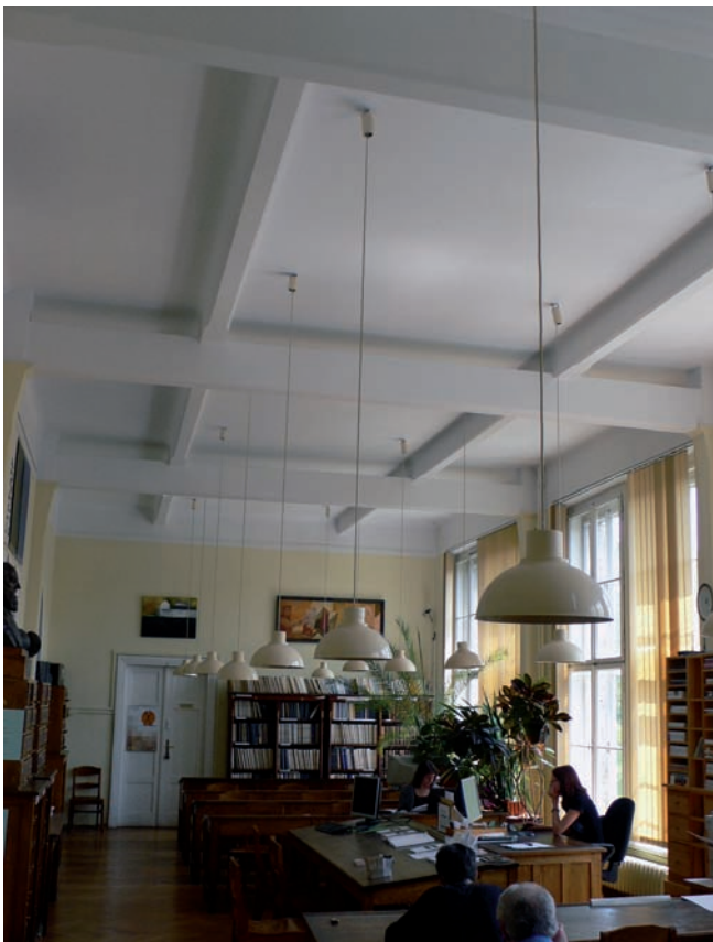
4. Kraków, Academy of Fine Arts Faculty of Industrial Design, reading room; floor structure as viewed from below: secondary beams resting on main beams which rest on posts adjacent to pillars between windows. Photo by W. Affelt
