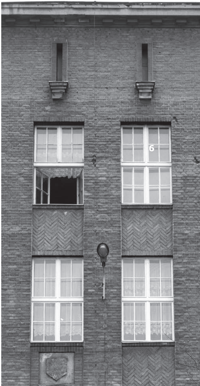
6. Detail of area between windows - School of Maritime Trade and Harbor Technology. Photo by the author
