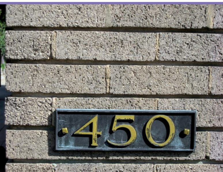
5. Meyer May House, Grand Rapids, 450 Madison Avenue SE, 1908-1909, Frank Lloyd Wright. A way of underlining the horizontal composition of Meyer May House using deep horizontal joints and filling vertical joints in external walls. A typical detail used by F.L. Wright in his prairie houses (photo by M. Czarnecki, 2007)
